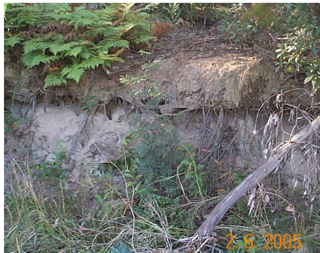
Photo 7 - Example of bank collapse of the Middle Creek Tributary
